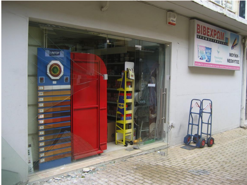
Photo 3.25. Damage at glass panes.
