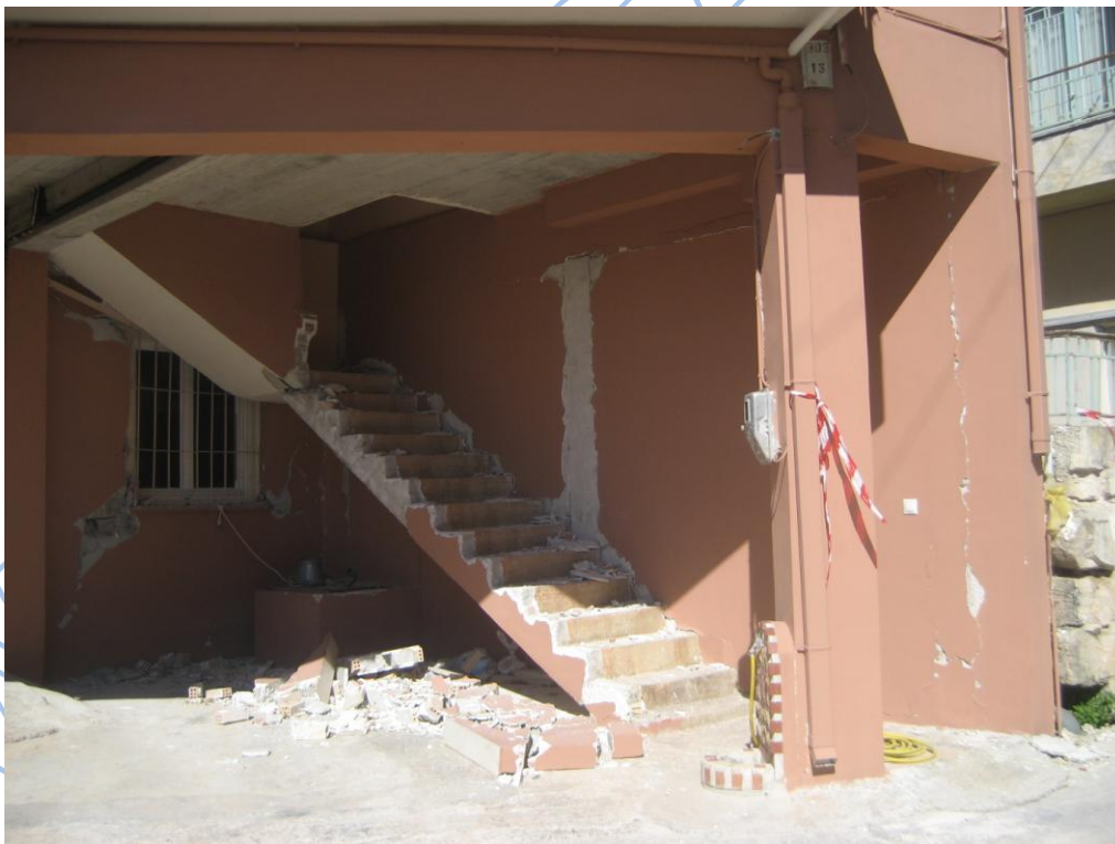
Photos 3.55, 3.56. Reinforced concrete building at the southern villages of Paliki peninsula as damaged during 26-1-2014 (up) and during 3-2-2014 (low) earthquakes.
