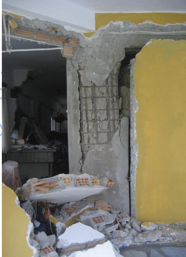
Photos 3.13, 3.14. Three storey building severely damaged in Livadi. Total collapse of
