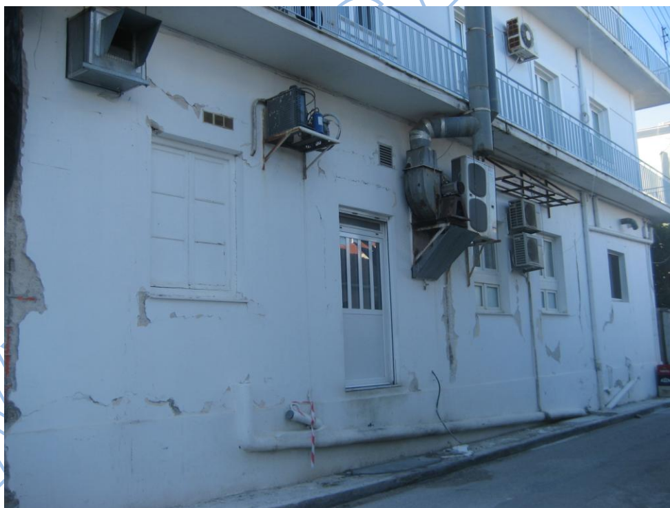
Photos 3.31, 3.32. Building in Argostoli as damaged during 26-1-2014 (up) and during 3-2-2014 (low) earthquakes.
