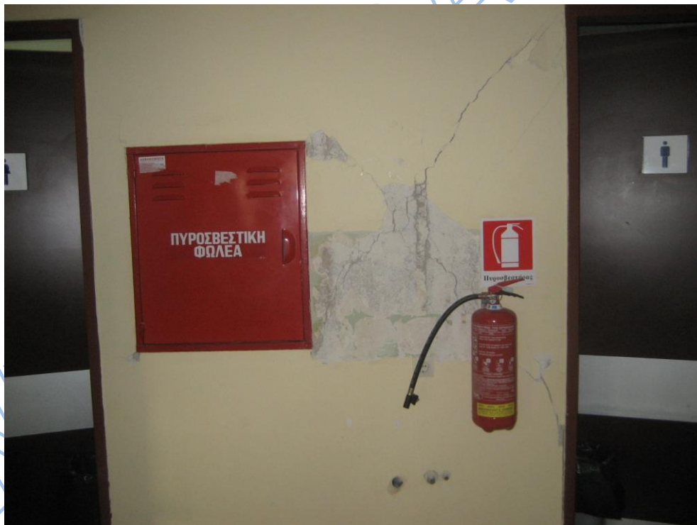
Photos 3.33, 3.34. Hospital in Argostoli as damaged during 26-1-2014 (up) and during 3-2-2014 (low) earthquakes.
