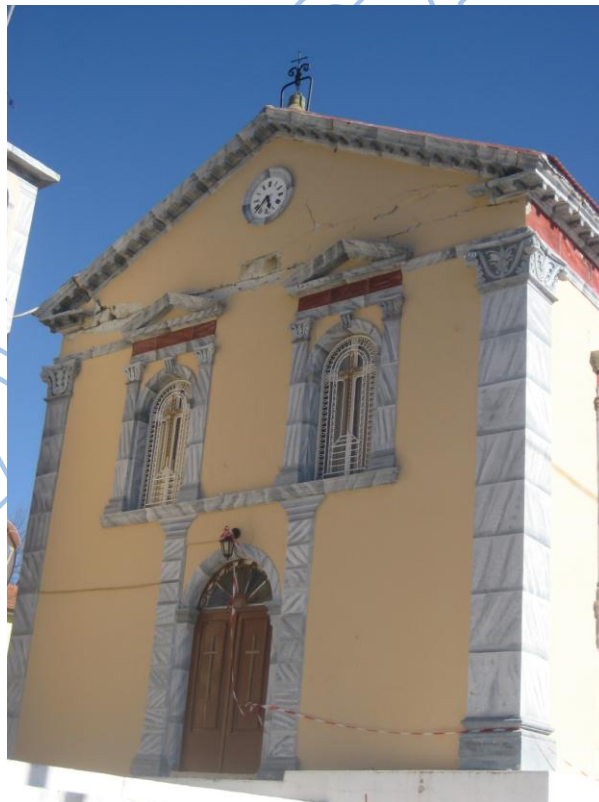
Photos 3.51, 3.52. Temple at the northern villages of Paliki peninsula as damaged during 26-1-2014 (up) and during 3-2-2014 (low) earthquakes.
