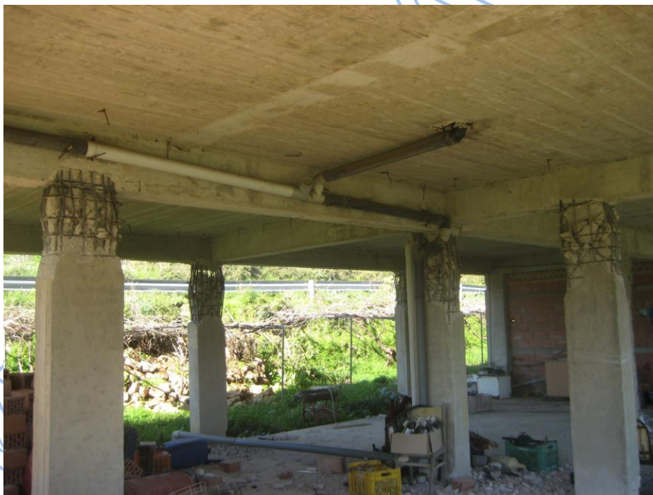
Photos 3.47, 3.48. Building on the way to Livadi as damaged during 3-2-2014 earthquake.
