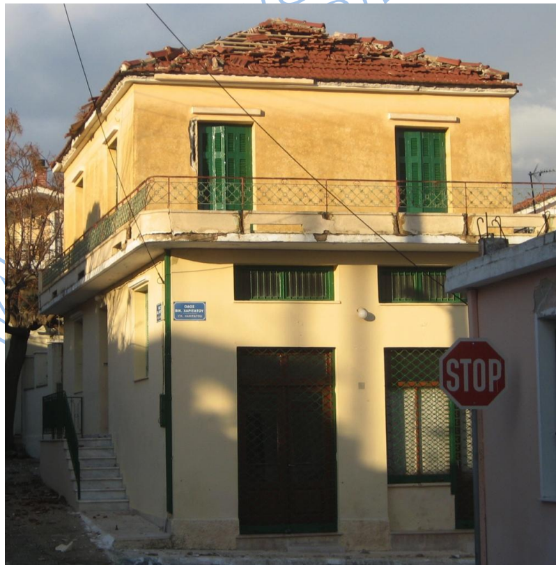
Photo 3.26. Damage on tile - roofs.
