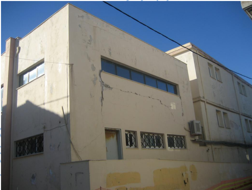
Photos 3.39, 3.40. School building in Lixouri as damaged during 26-1-2014 (up) and during 3-2-2014 (low) earthquakes.
