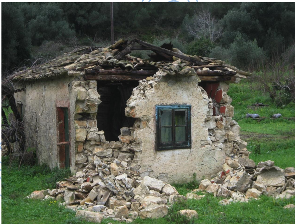
Photos 3.3, 3.4. Partial collapses of masonry buildings of secondary use.
