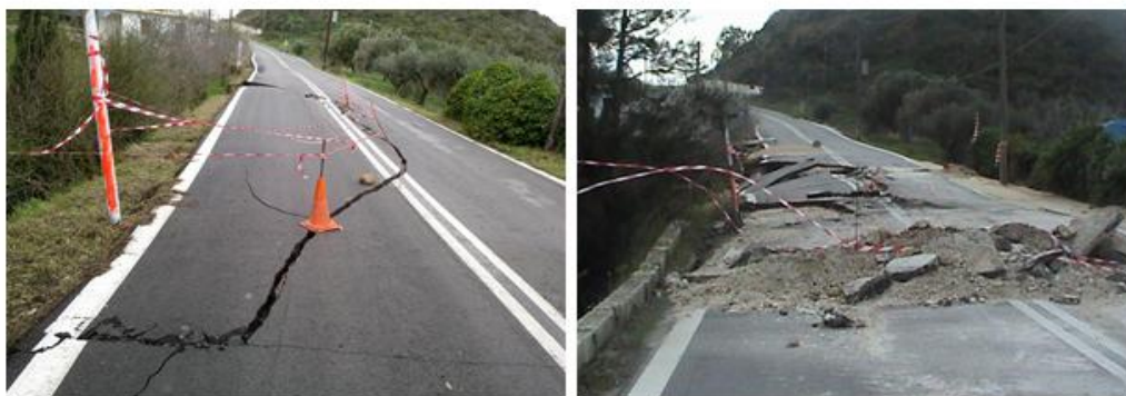
Figure 2.12. Road connecting Chavriata and Vouni villages. Left: Circular type of sliding observed after the first earthquake. Right: Embankment failure after the second earthquake inducing total road damage.
