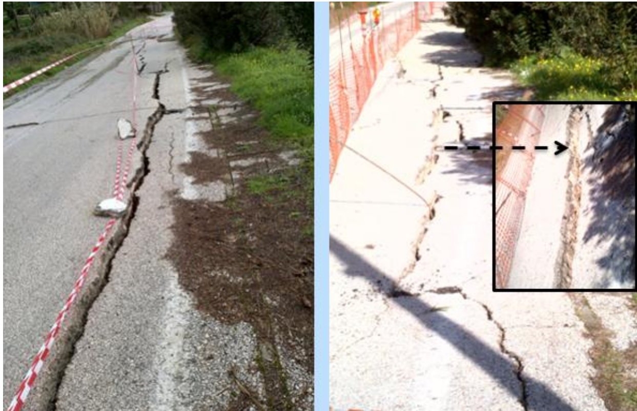
Figure 2.13. Cracks and embankment settlement recorded at the road network between Agios Dimitrios and Livadi villages ( 38.238103^{\circ}\text{N} , 20.428973^{\circ}\text{E} ) induced by the first (left) and the second (right) earthquake.
