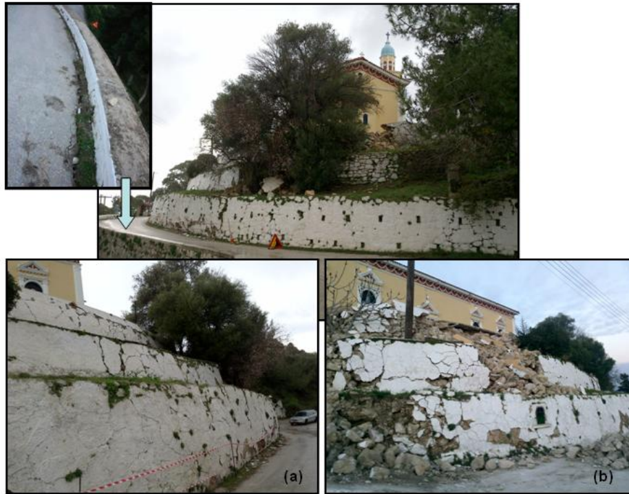
Figure 2.9. Major failure of a three-level stone masonry retaining wall supporting the foundation soil of a church in Chavriata village (38.182677° N, 20.387261° E): (a) Extensive cracks observed following the first earthquake of 26/01/2014 (b) total collapse of the wall following the second strong earthquake of 03/02/2014.
