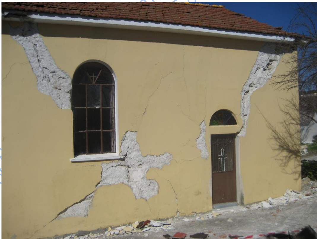
Photos 3.59, 3.60. Temple at the southern villages of Paliki peninsula as damaged during 26-1-2014 (up) and during 3-2-2014 (low) earthquakes.
