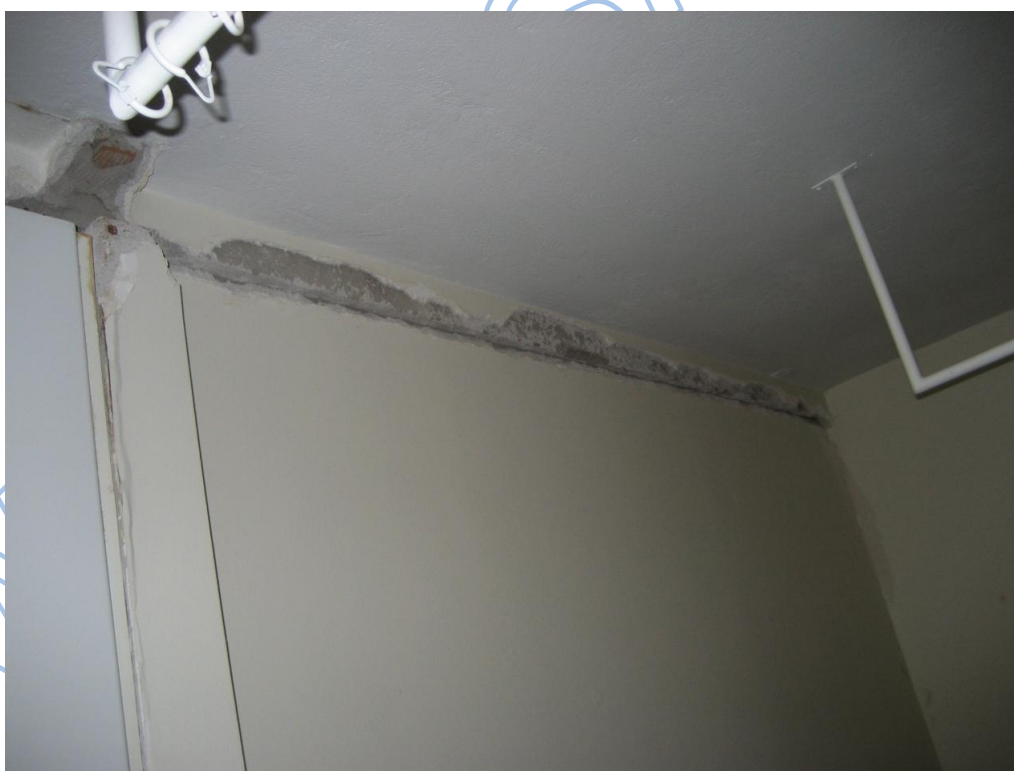
Photos 3.7, 3.8. Cracks between structural element and infill walls of the elderly people nursery (up) and the hospital (bottom) at Argostoli. These buildings were temporarily abandoned.
