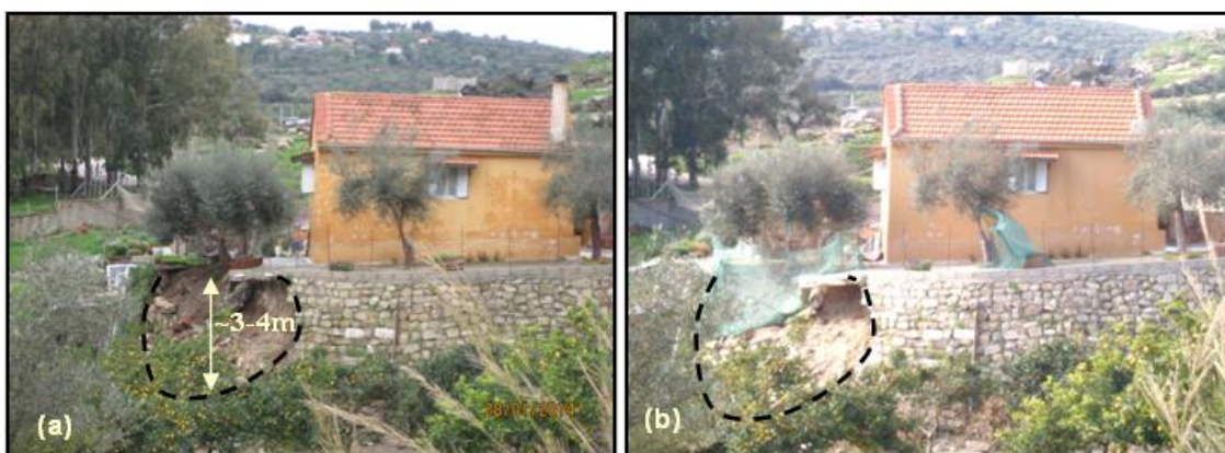
Figure 2.10. Single-storey building close to Kouvalata village (38.234484° N, 20.419554° E): (a) Failure of the stone masonry retaining wall followed by local landslide of the supporting foundation soil after the first earthquake of 26/01/2014, (b) Further deployment of the failure surface after the second earthquake of 03/02/2014.
