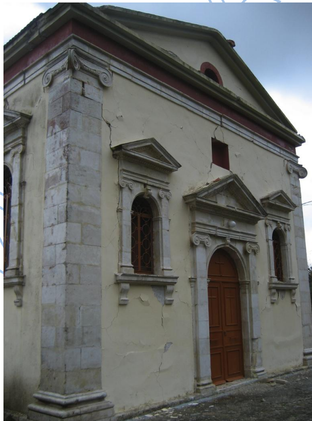
Photos 3.23, 3.24. Cultural heritage masonry building and temple, with damage, at the center of Paliki peninsula.
