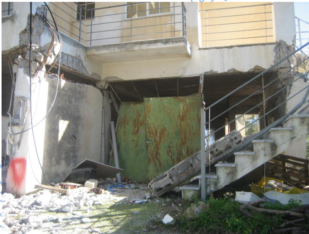
Photos 3.43, 3.44. Building in Agios Dimitrios as damaged during 26-1-2014 (up) and during 3-2-2014 (low) earthquakes.
