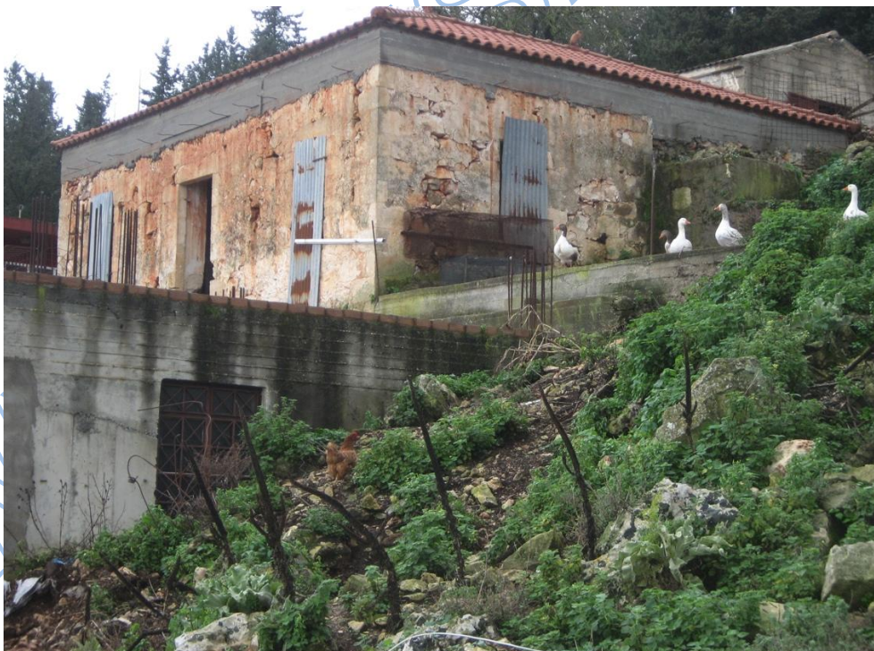
Photos 3.1, 3.2. Two neighbor masonry buildings at the villages. The building with strong R/C ties at top had no damage.
