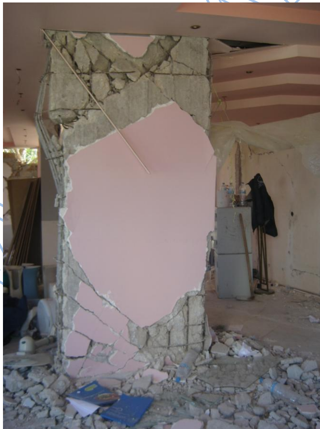
Photos 3.41, 3.42. Building in Lixouri as damaged during 3-2-2014 earthquake.
