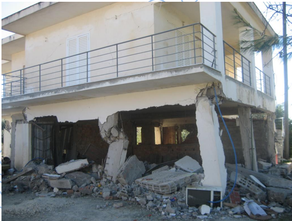
Photos 3.45, 3.46. Building in Agios Dimitrios as damaged during 26-1-2014 (up) and during 3-2-2014 (low) earthquakes.
