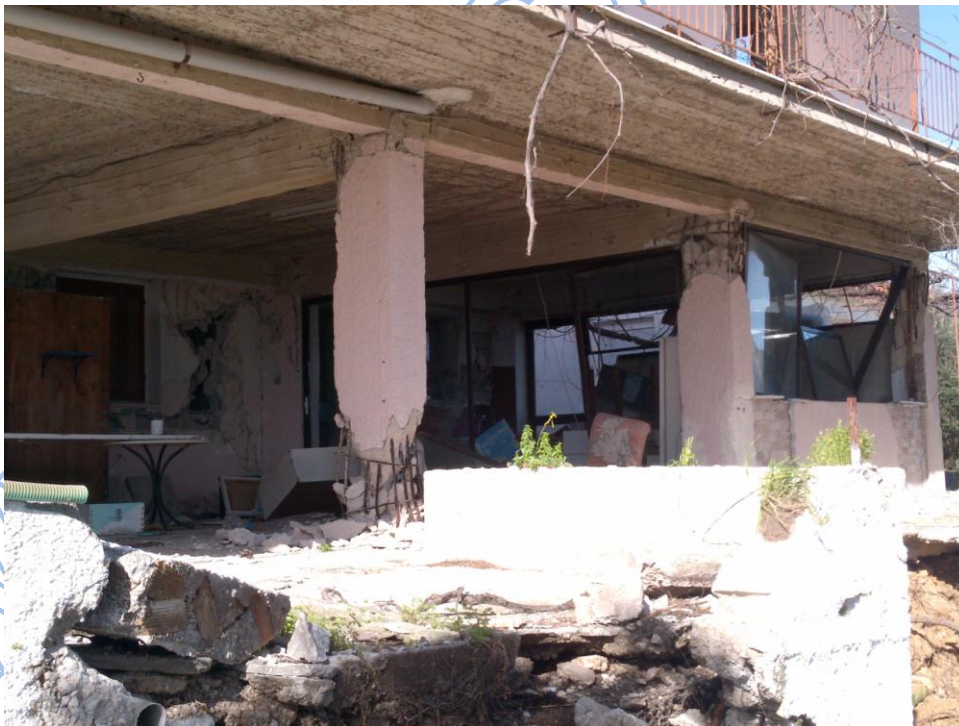
Photos 3.49, 3.50. Building on the way to Livadi as damaged during 26-1-2014 (up) and during 3-2-2014 (low) earthquakes.
