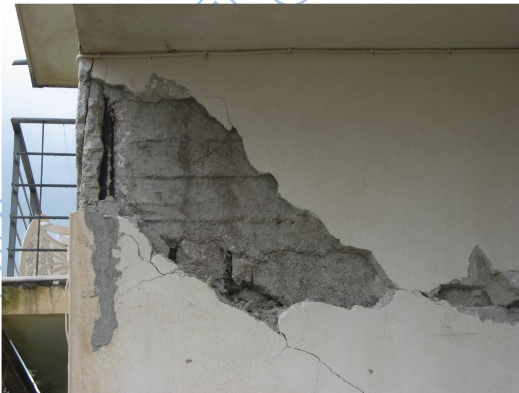
Photos 3.11, 3.12. Damage at a two storey building in Agios Dimitrios.
