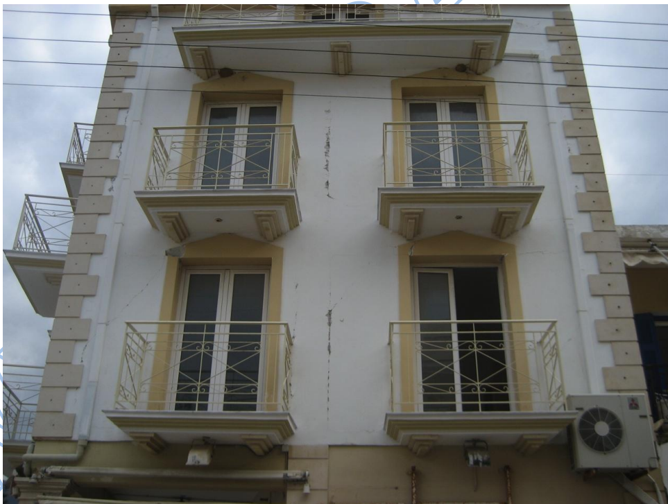
Photos 3.5, 3.6. Multistory buildings with detachment of infill walls from the R/C frames. No damage to the structural elements were observed.
