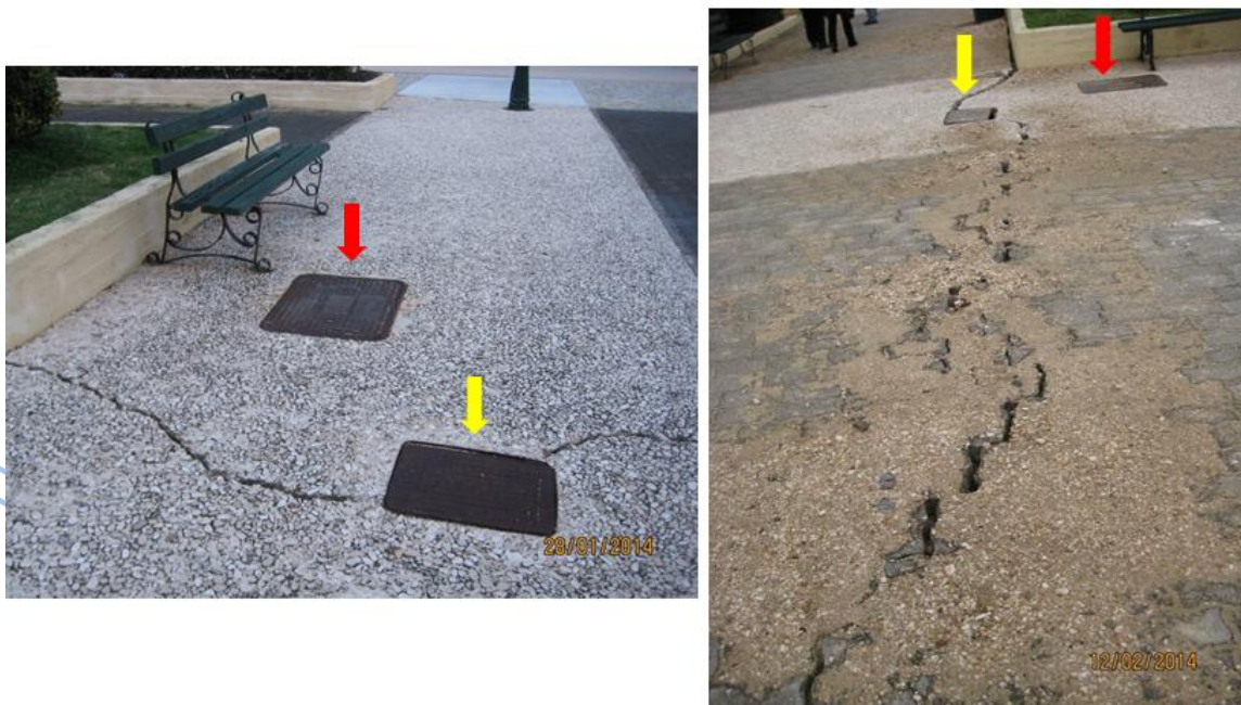
Figure 2.19. Indicative case of the extensive liquefaction ejecta induced by the second earthquake of 03/02/2014 (right) compared to the first earthquake of 26/01/2014. Photos taken at the same point form a different angle.
