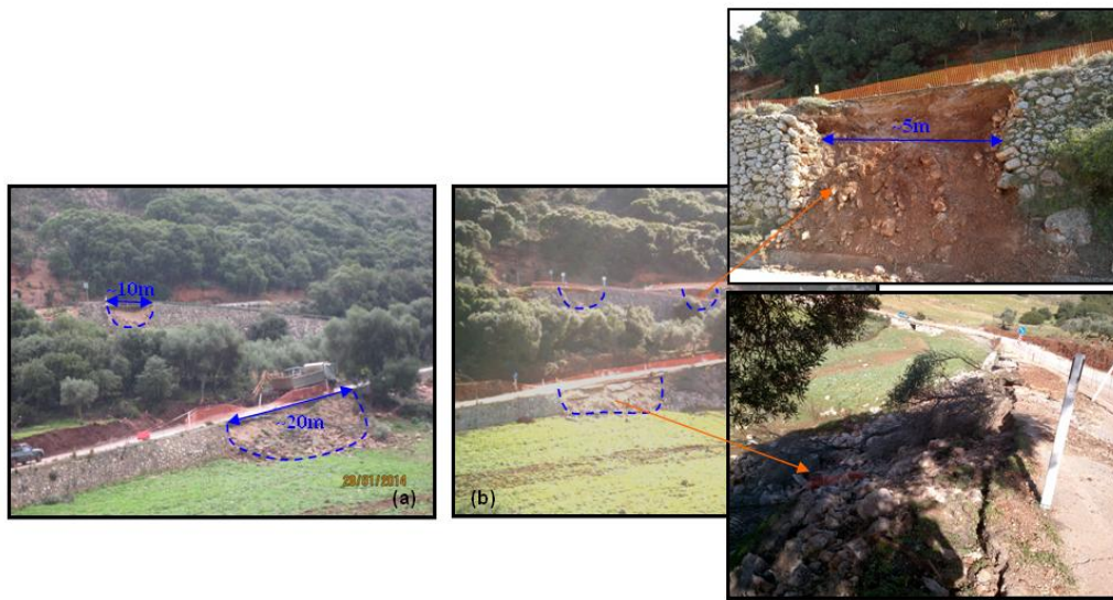
Figure 2.8. (a) Extensive failure of a stone masonry retaining wall followed by road embankment settlement close to Atheras Village ( 38.293224^{\circ} N, 20.45217^{\circ} E) after the first earthquake of 26/01/2014. (b) Additional failure surface at a third location of the wall induced by the second strong earthquake of 03/02/2014.
