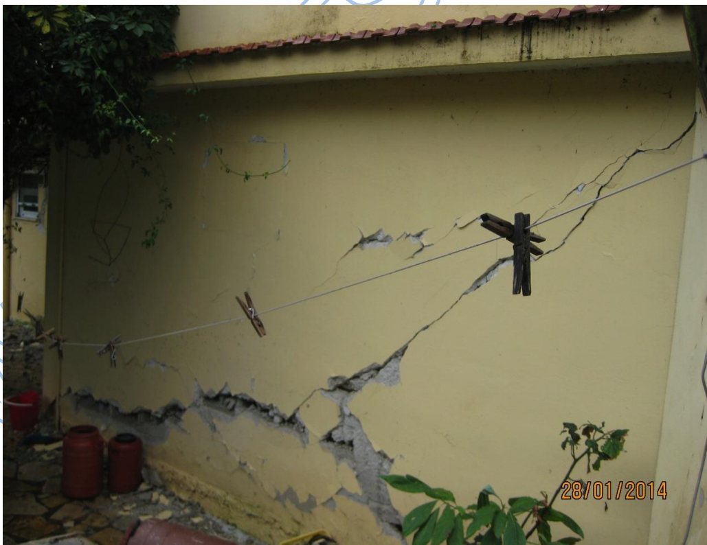
Photos 3.15, 3.16. Two storey building with damage, at the Northern road from Lixouri.
