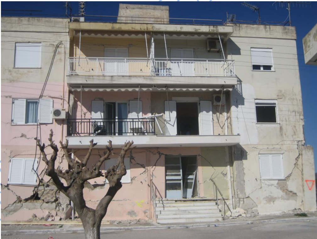
Photos 3.37, 3.38. Labor houses in Lixouri as damaged during 26-1-2014 (up) and during 3-2-2014 (low) earthquakes.
