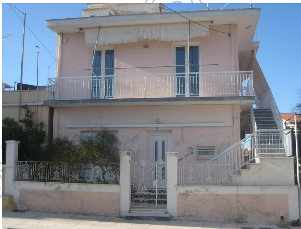
Photos 3.29, 3.30. Building in Argostoli as damaged during 26-1-2014 (up) and during 3-2-2014 (low) earthquakes.
