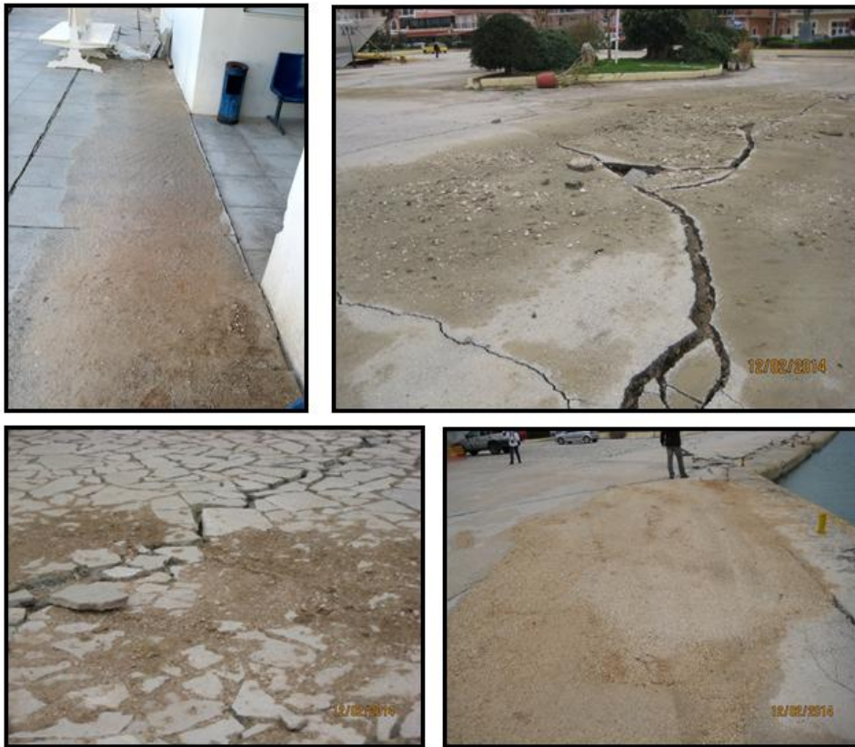
Figure 2.18. Typical liquefaction ejecta recorded along Lixouri port.
