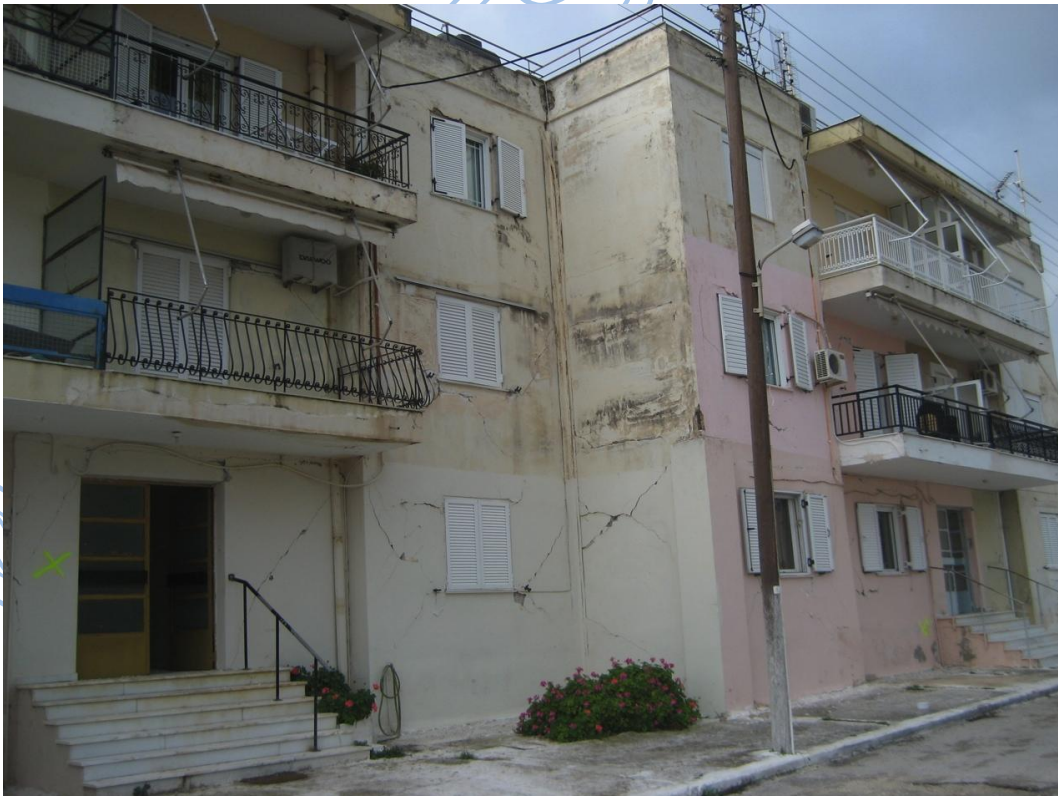
Photos 3.9, 3.10. Damage at the Labour houses at Lixouri.
